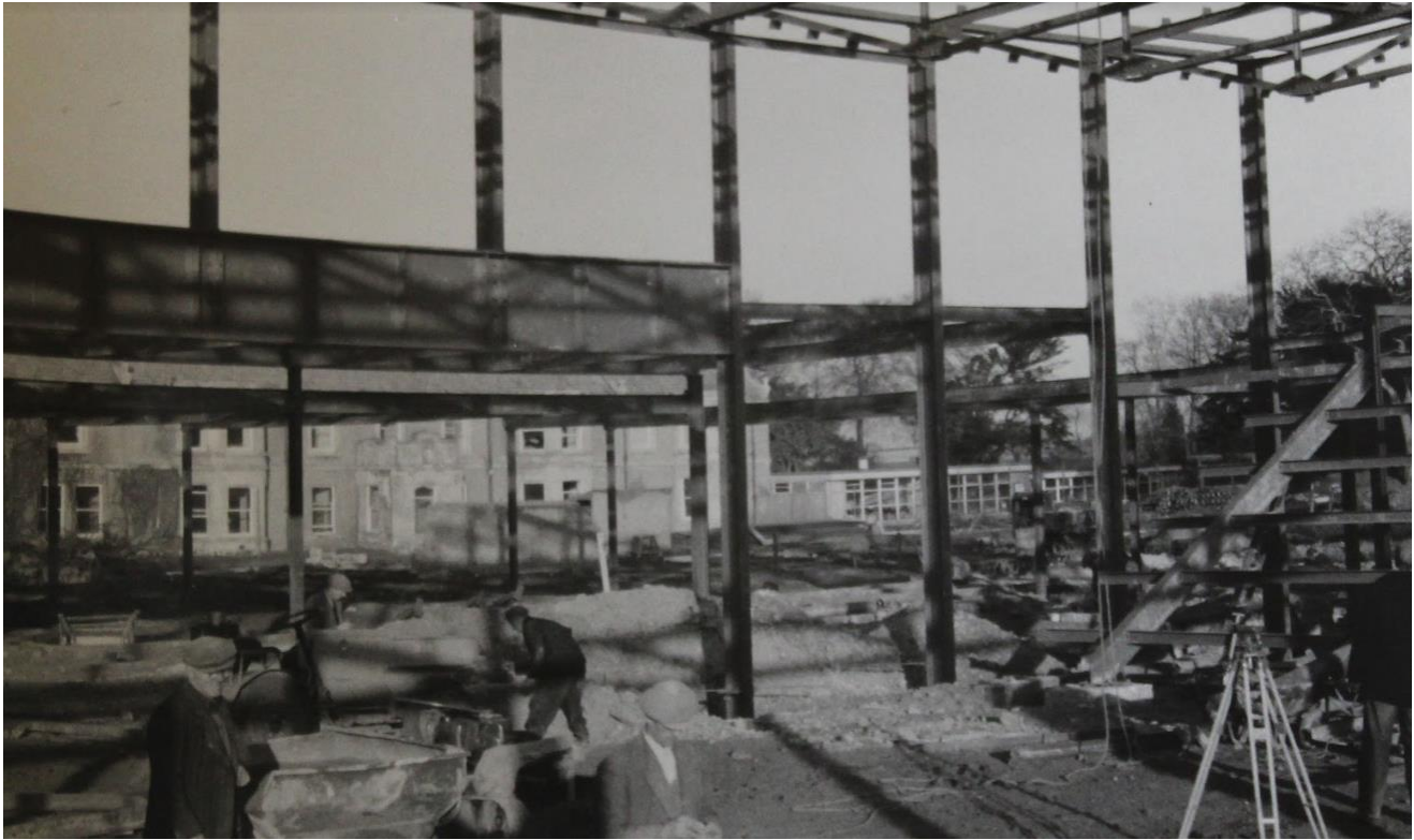
The main hall (note the steelwork for the ramp on the right) The days before PPE...
